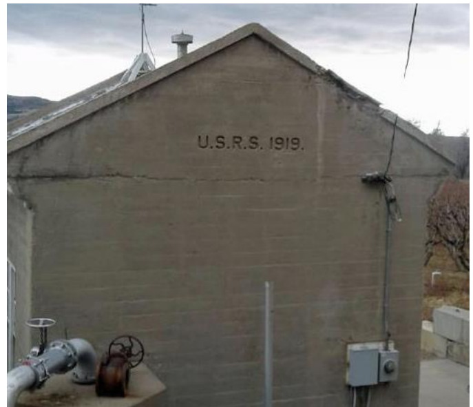
U.S.R.S. (United States Reclamation Service) and the construction year, 1919, are still visible on the Stub Pumping Plant's 100 year old building in this recent photo.
