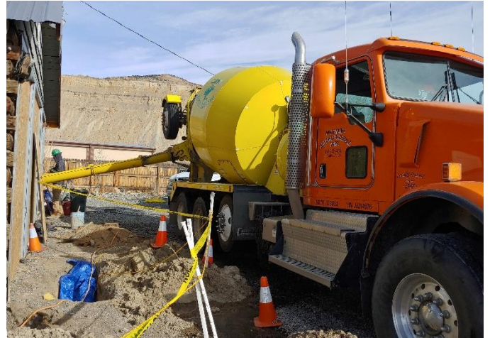
Whitewater Building Materials poured concrete for the inside floor the third week of January.
